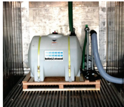
Installation at O'Hare Airport in Chicago
